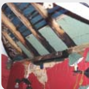
Incident investigation – the effects of an LPG explosion
