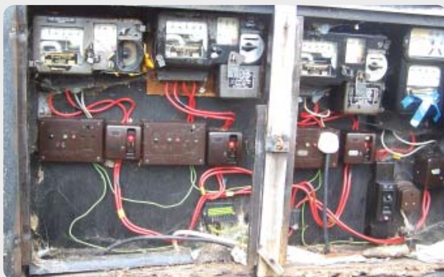
Ingress of water and exposed live conductors make this intake on a caravan site dangerous. Residents also had to feed their meters here.
