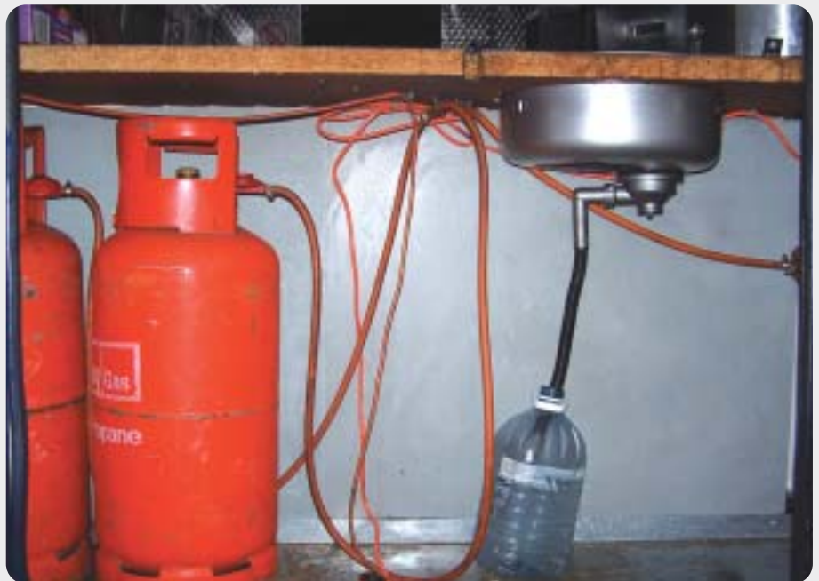
Sub standard LPG installation in a mobile trader's vehicle. Solid copper piping should be used throughout.
